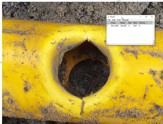
Fig. 3. Example of a photo taken during the excavation of a third party damage
